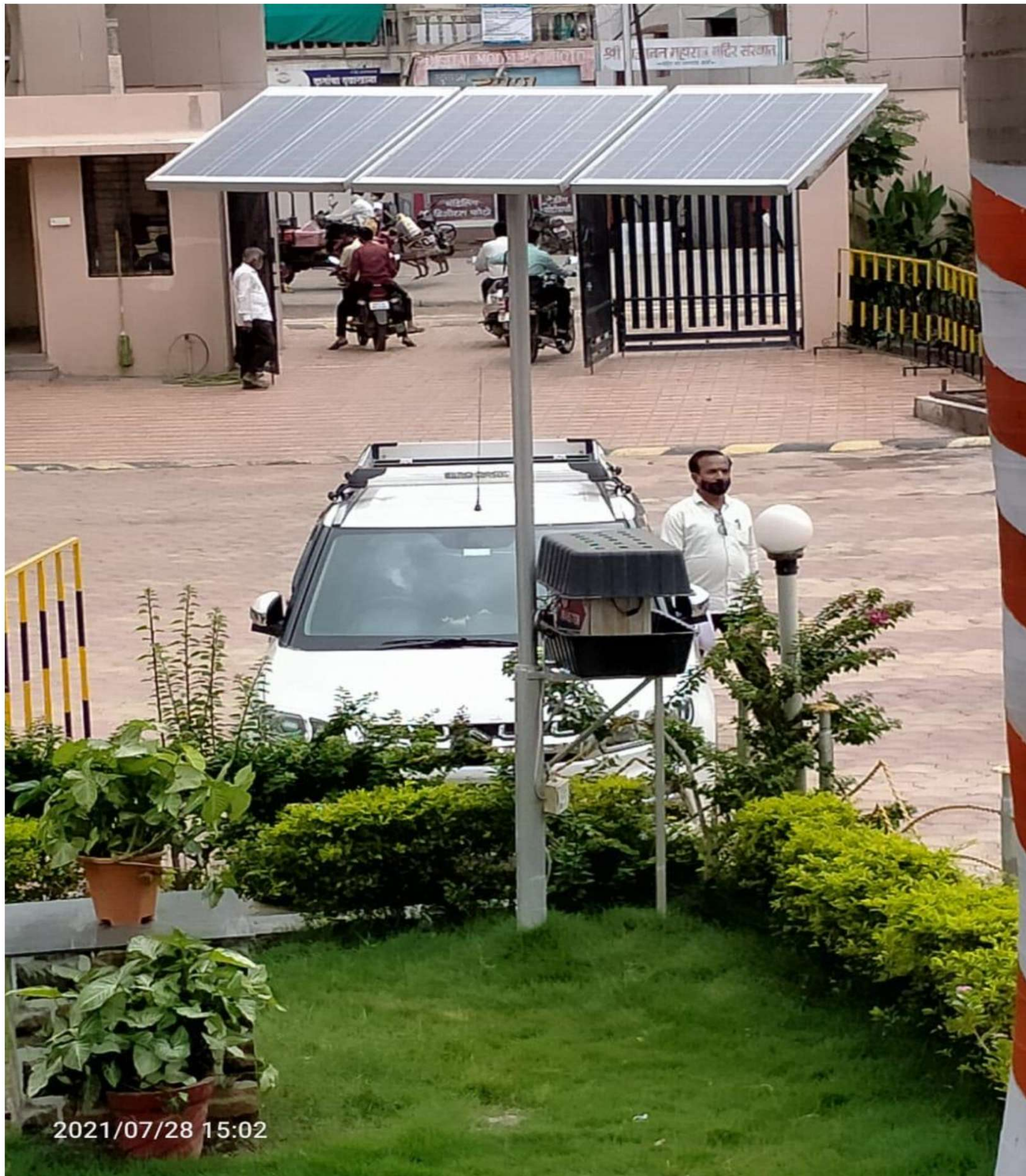
Fig. Solar lights installed near Bhausahab Statue
